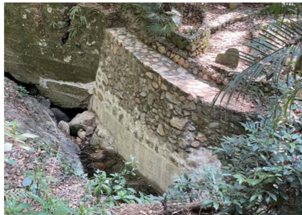
Unregistered slope in Orchid Haven near the Entrance
